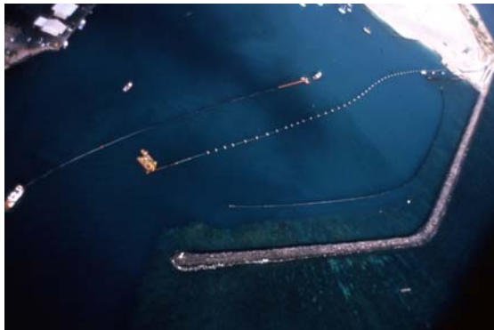
Figure 3. Deployment of a 1 m (40”) diameter CWP (photo courtesy of Makai Ocean Engineering, Inc.)
